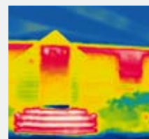
Building: Heat Loss
