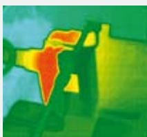
Motor: Bearing Problem
